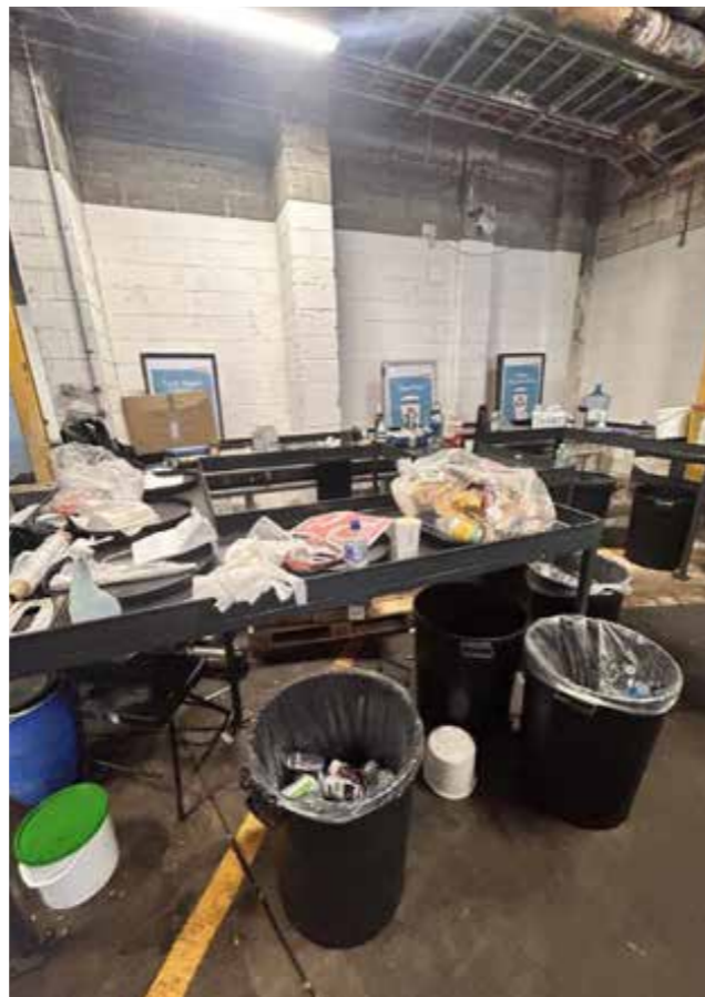
We are working with our colleagues in the wider industry to tackle on board waste recycling, we're learning from best practice, such as this waste recycling facility in Euston, London
